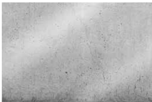
Nr.: 453 Cracked Concrete
